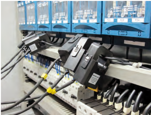
Measurement of power supply
